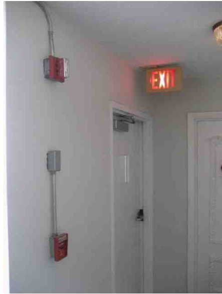
pull station, strobe, siren, lit emergency exit
