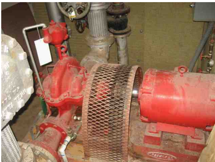
water booster / fire pump (un-finished)
