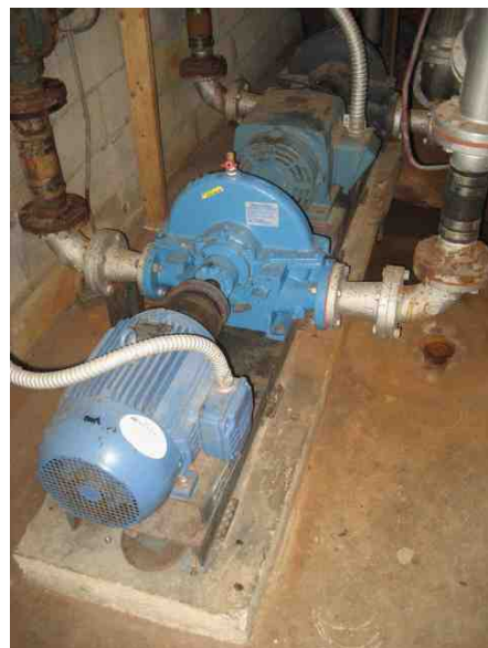
domestic water pumps (un-finished)
