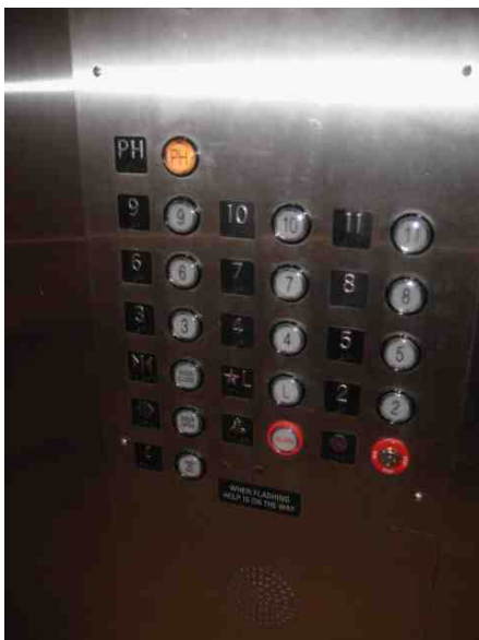
12 stop elevator panel
