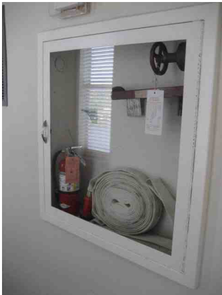
fire hose / extinguisher
