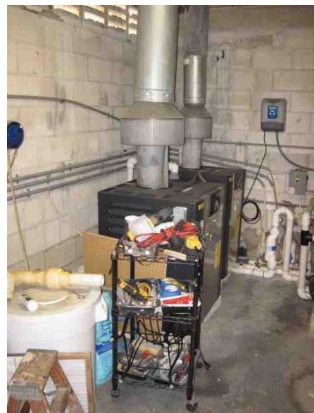
pool equipment / heaters
