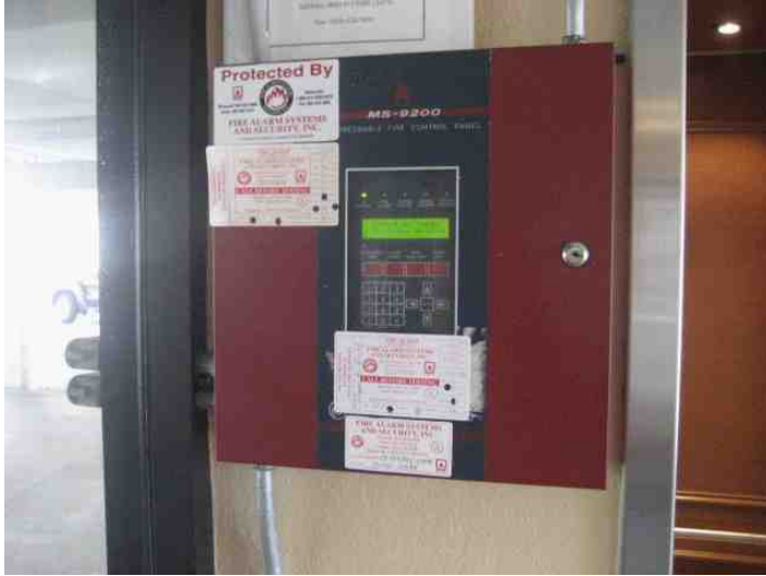
master fire alarm panel
