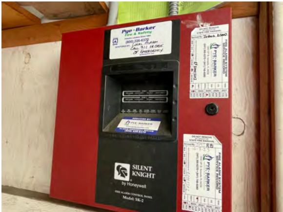
GENERAL VIEW OF FIRE ALARM PANEL
