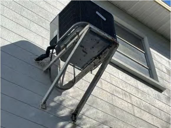
VIEW OF HVAC EQUIPMENT
